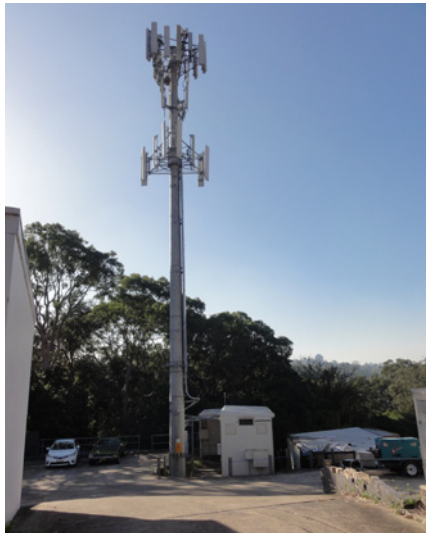
Telecommunication tower and station on site
